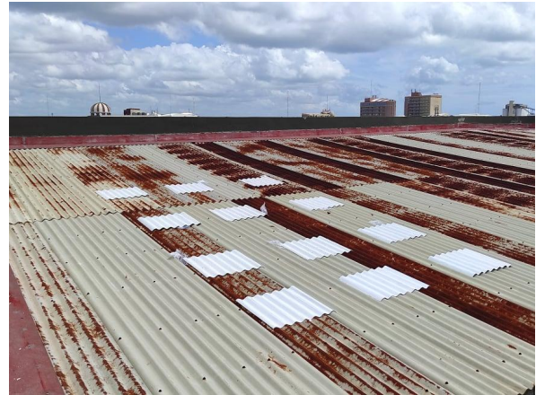
Figure 1. Experimental set-up of roof sheets.
