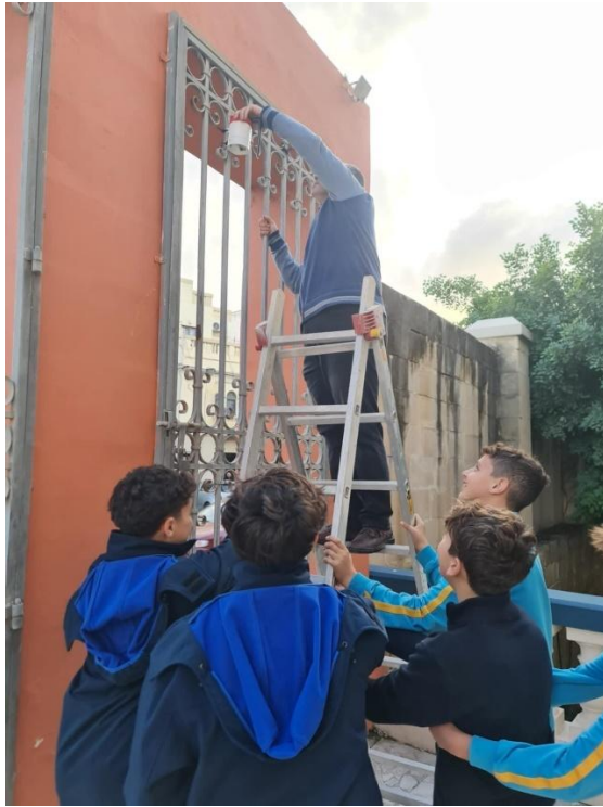
Figure 1: Tube installed in the school premises
