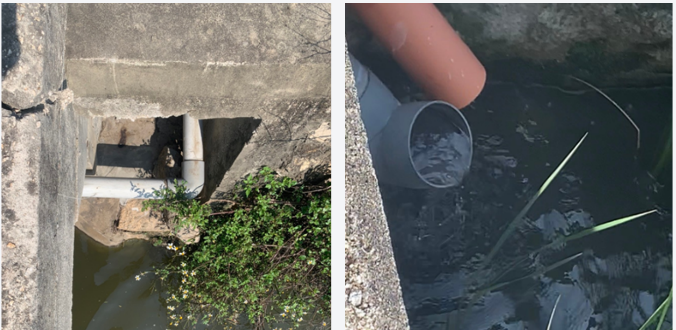
▲Fig13: Water pipes connecting to the reservoir
