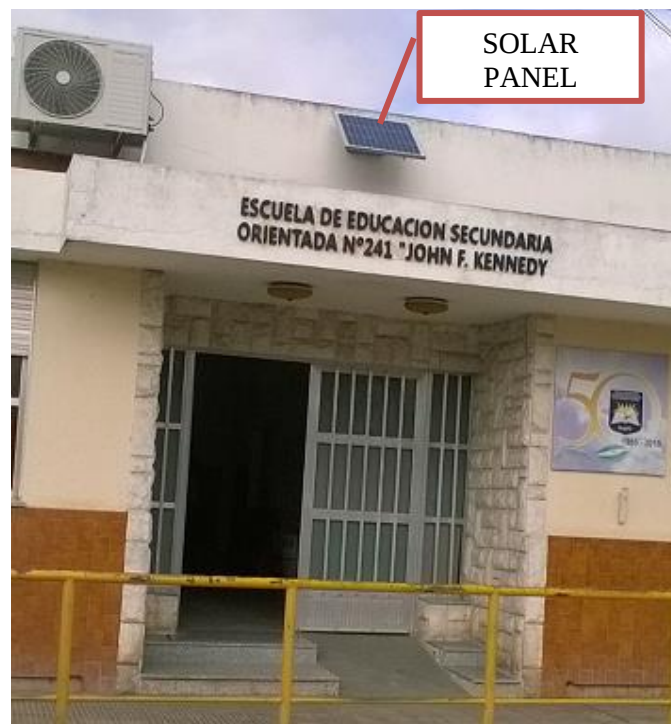
Figure 2: View of the front of the EESO 241 where the solar panel is installed
